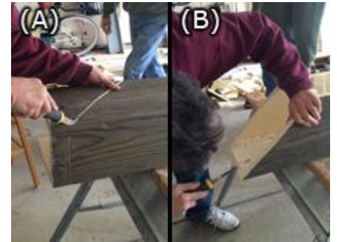
12. Cutting Beam (a) Cut one side then cut the other side. (b) Flip beam over, cut bottom. When finished, trim inside ends for a snug fit.
