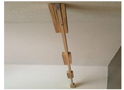
9. Wood blocks spaced every 3-4 feet on support structure will provide a snug fit when beam is raised into place.
