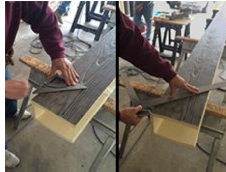
11. Using angle of ceiling, draw line onto beam sides and bottom, score with blade.
