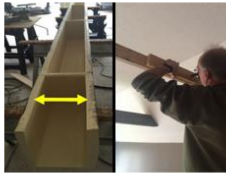
8. Measure inside width of faux beam . Use additional wood blocks spaced every 3-4 feet to build out support structure. To snugly fit the interior of the faux beam.
